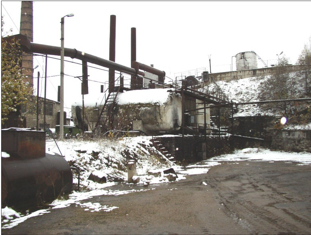
Photo 4000-3. Shale oil boilers; 15.10.2002
