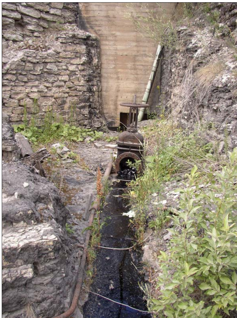
Photo 4000-5. Slowly leaking naphtha bitumen close to underground tank No 5; 21.07.2006
