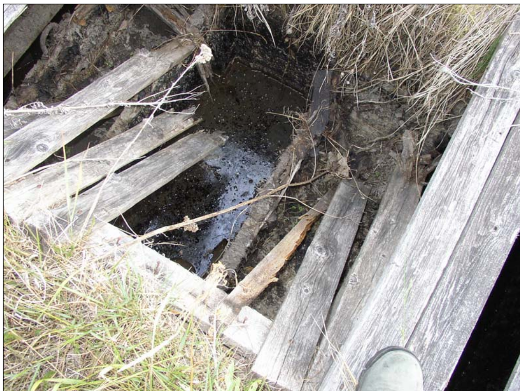
Photo 4000-10. Same oil separator (view take closer); 21.07.2006 visible oil products residue in separator
