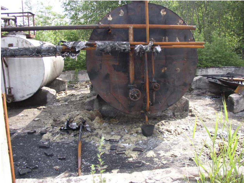
Photo 5703. Aboveground fuel tank 2003.a
