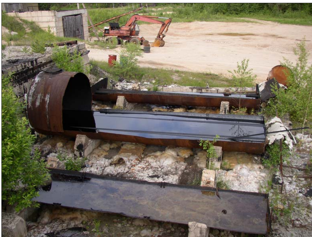
Photo 6600-2. View to open oil shale oil tanks (16.06.2003)
