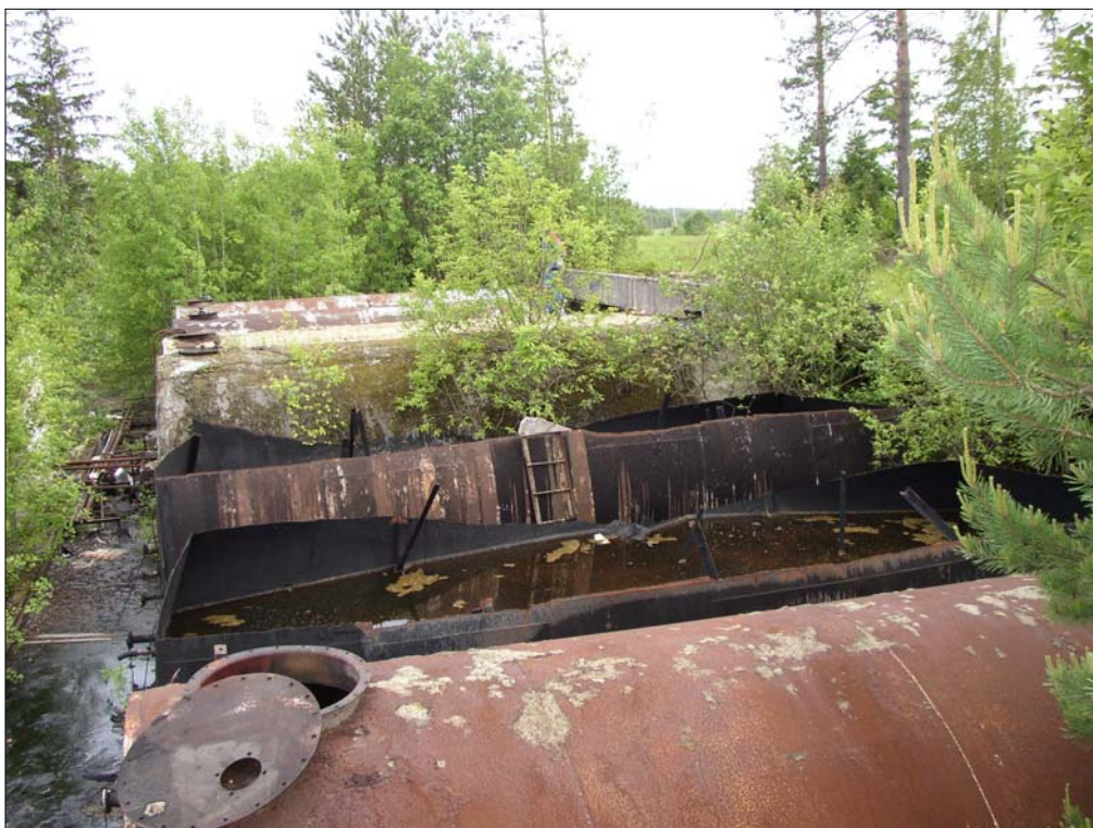
Photo 6600-1. View to open naphtha bitumen tanks (16.06.2003)
