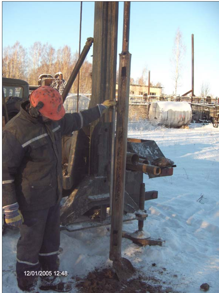
Photo 6521. Bore hole 6521 – oily layer between 2,5-3,4 m
