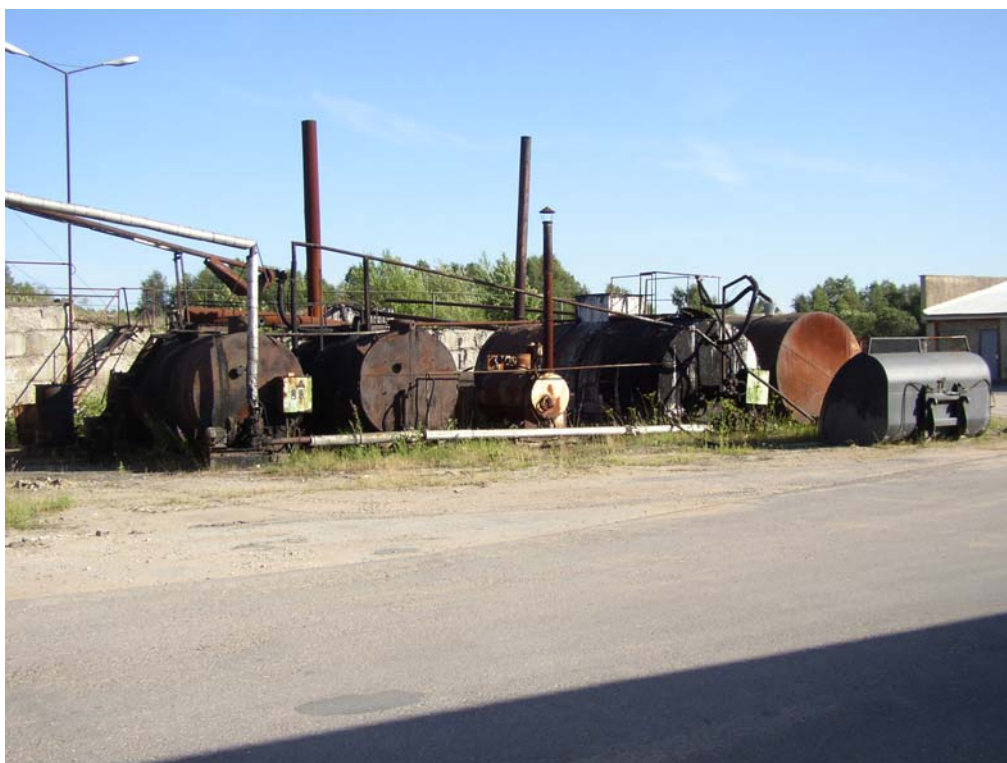
Photo 4700-3. View to the tank and boilers area; photo 12.07.2006
