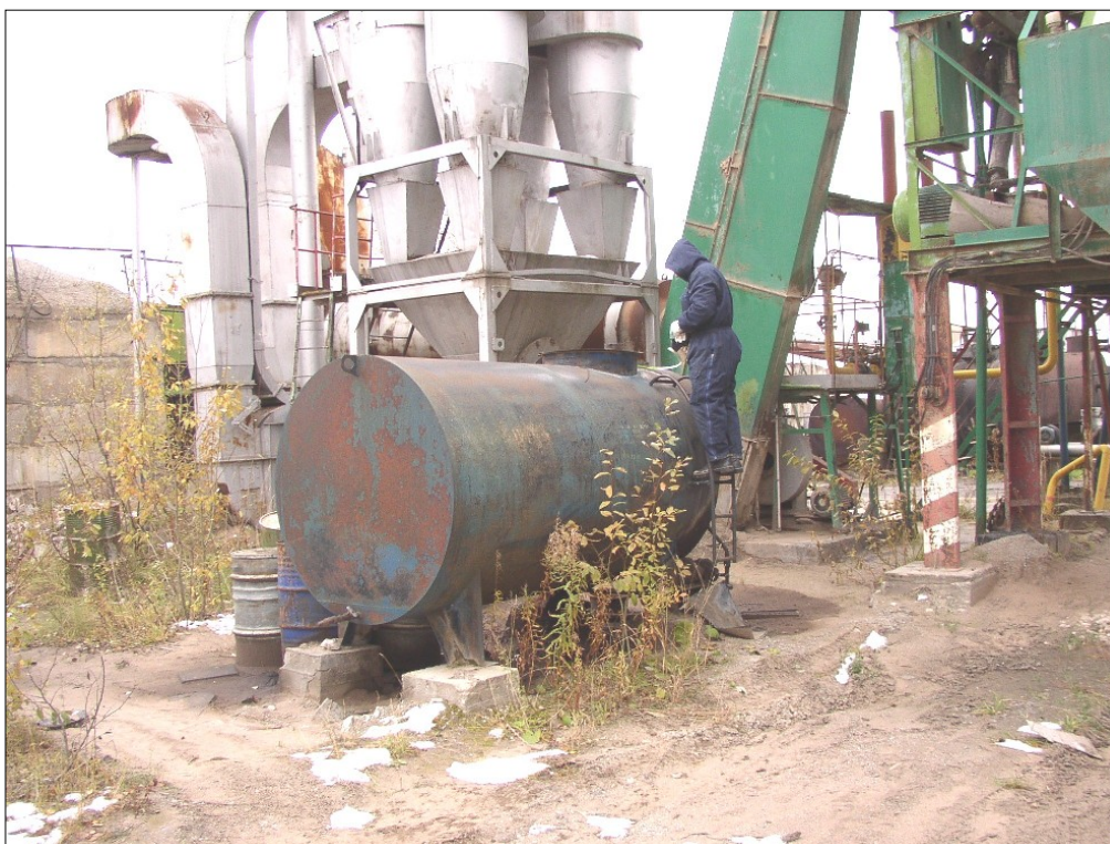
Photo 4700-2. View to still use tank of fuel; photo 15.10.2002
