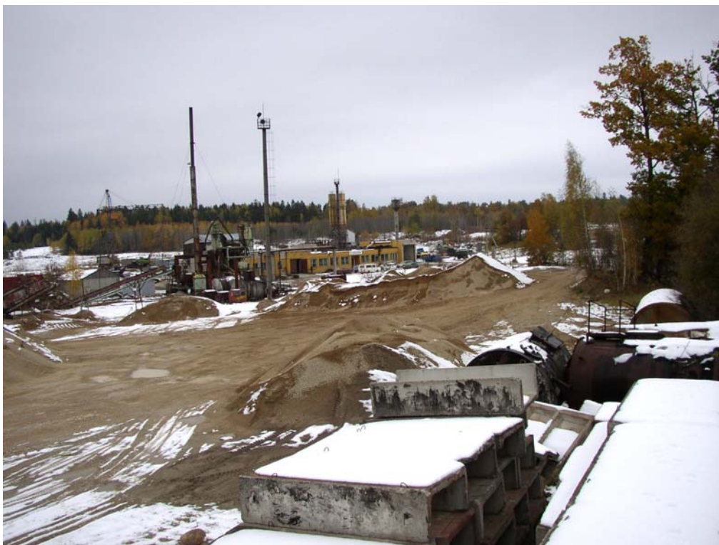
Photo 4500-1. View to the asphalt mixing plant from South-West; photo 16.10.2002
