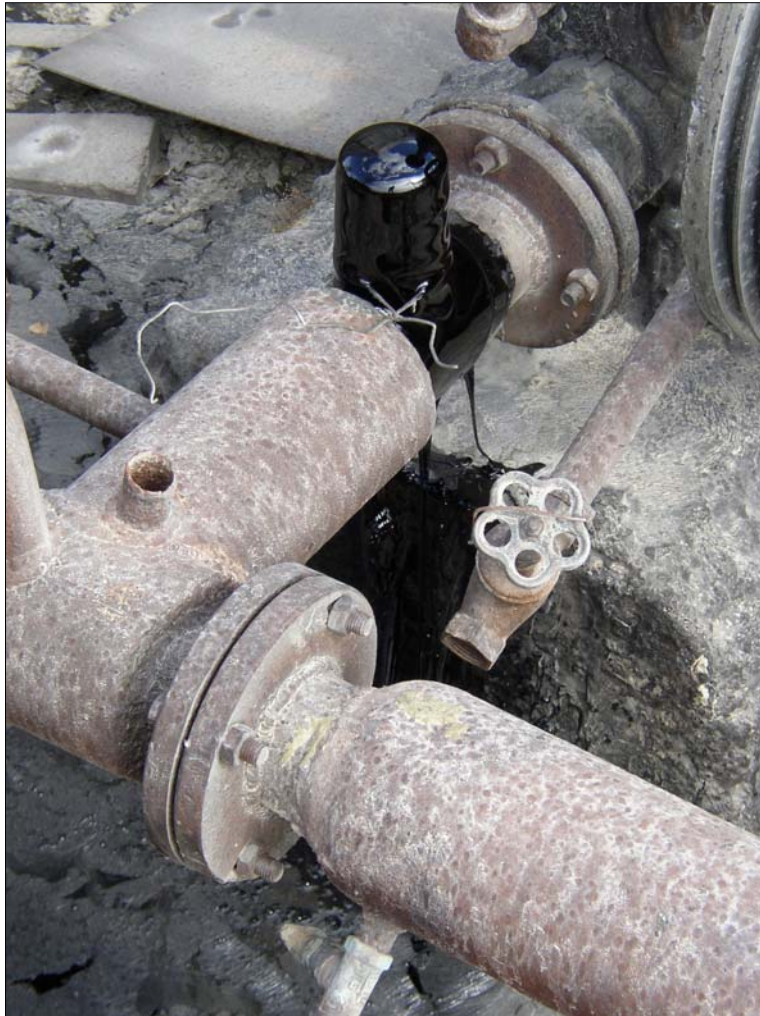
Photo 4500-6. View to leaking pipes closer; photo 17.07.2006
