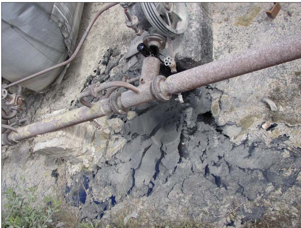
Photo 4500-5. View to the underneath pool of tank area; photo 17.07.2006 From open pipes leaks bitumen residue
