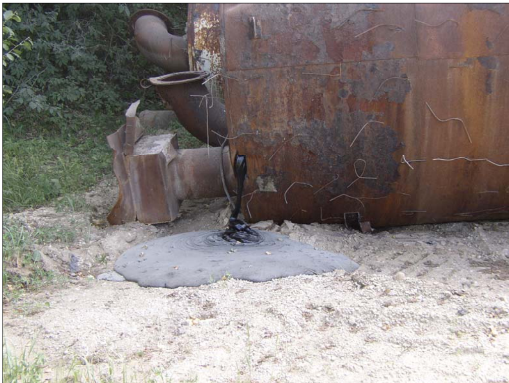
Photo 4500-4. Leaking tank close to the bore hole 4501; photo 17.07.2006 From hole in the tank leaks bitumen residue
