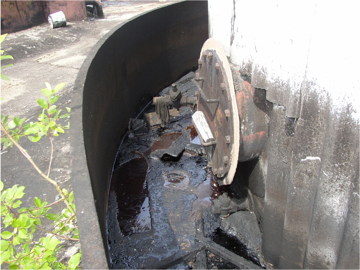
Photo 3 Inside steel barrier remained black oil and shale oil residuals
