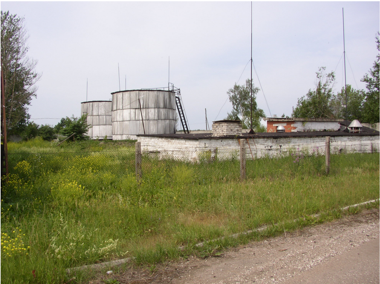
Photo 4 Two a'180 tons tanks and old pumping house with one 60 tons tank in cellar
