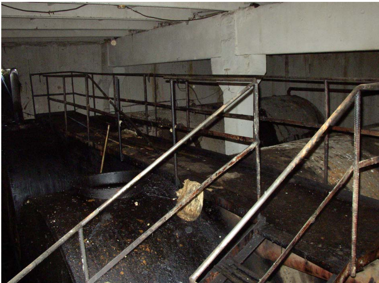
Photo 4 Two black oil tanks in cellar
