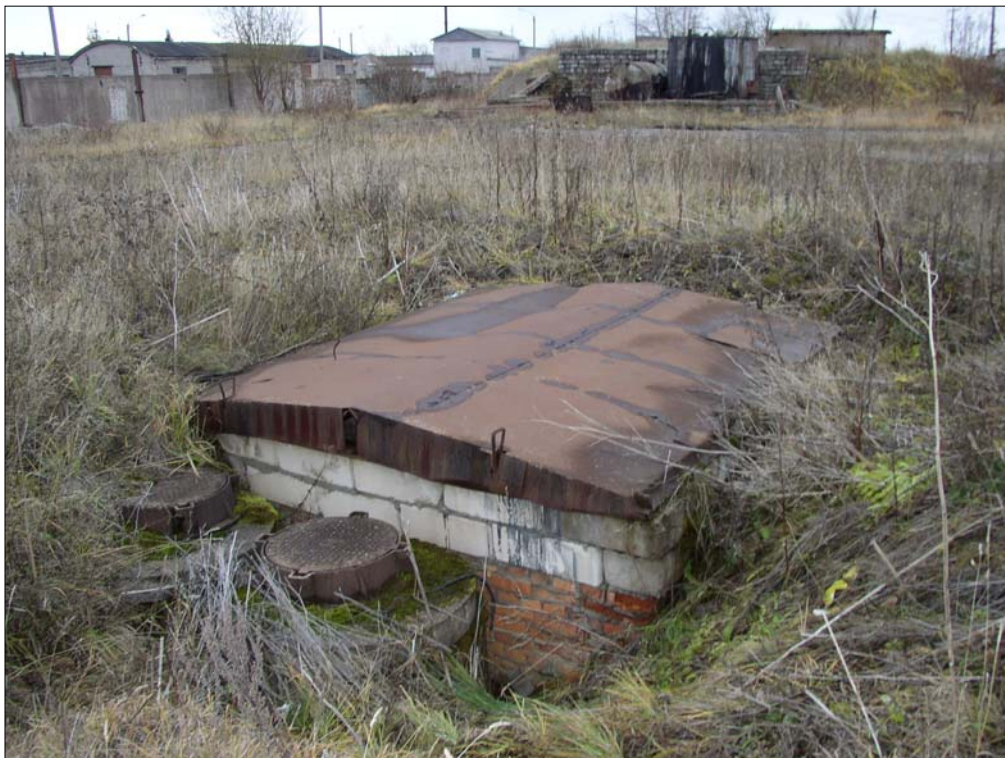
Photo 2900-8. View to the not working oil separator; photo 29.10.2002
