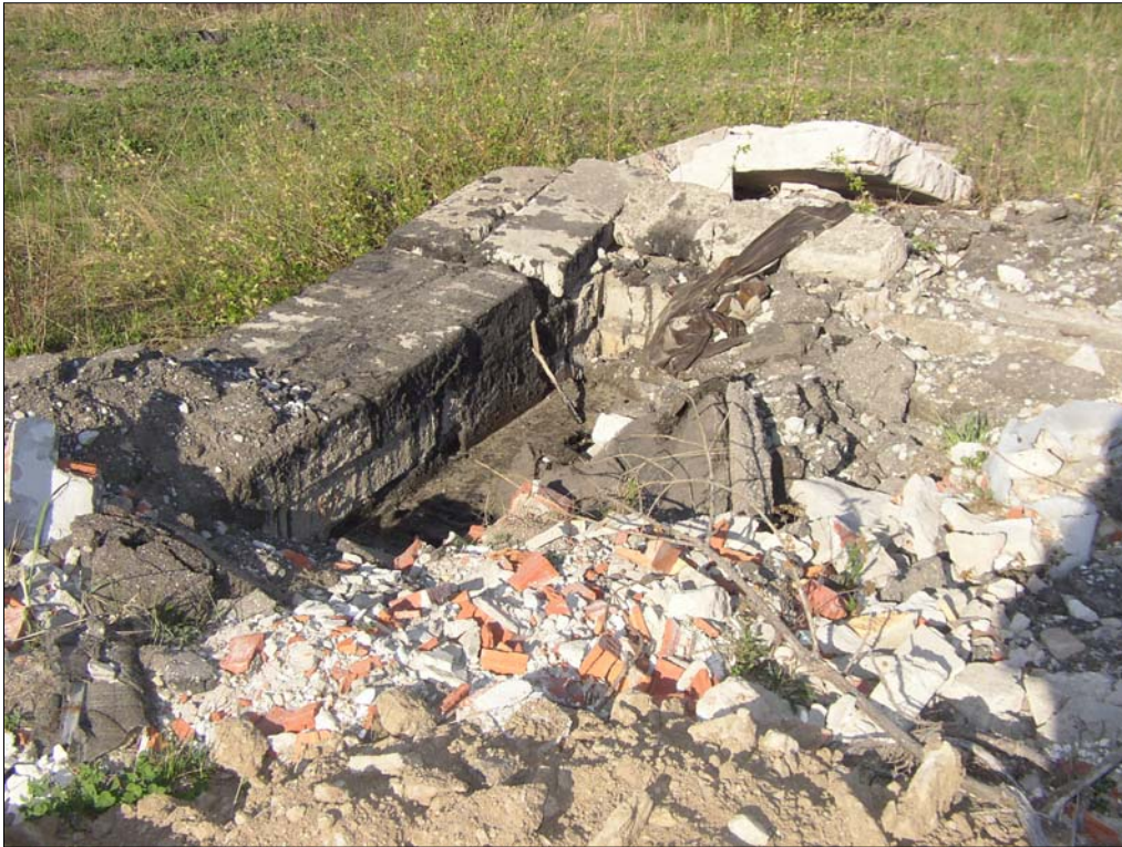
Photo 2900-7. View to north-east corner of former tank area, free bitumen inside basement walls; photo 27.04.2006
