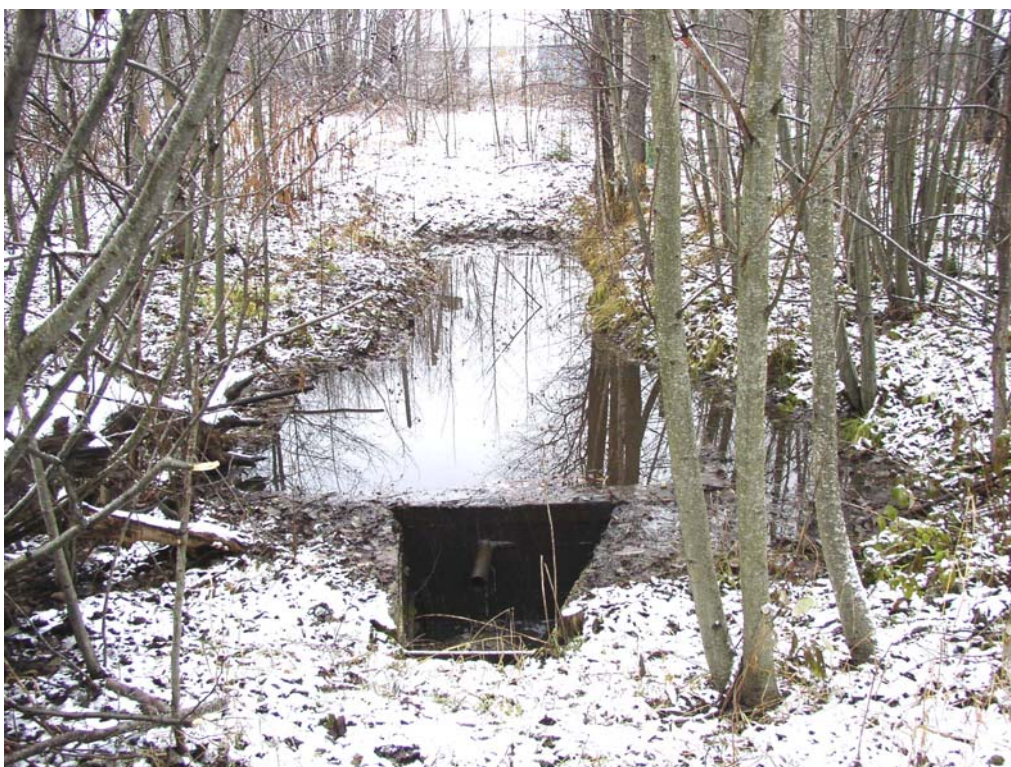
Photo 2500-3. View to the not working primitive oil separator (12), which is filled up to the top; in front the outflow pipe to ditch; photo 30.10.2002
