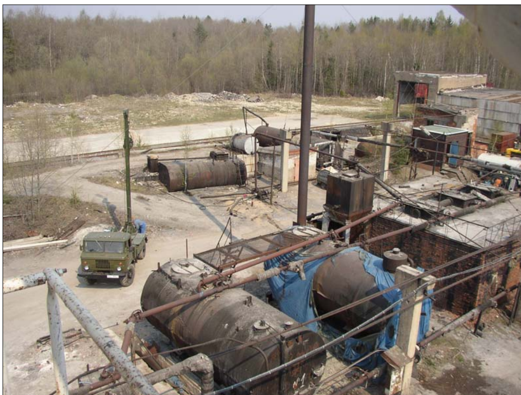
Photo 2500-1. View to working part of Ahtme mnt 88 ABT; in front 2 boilers
