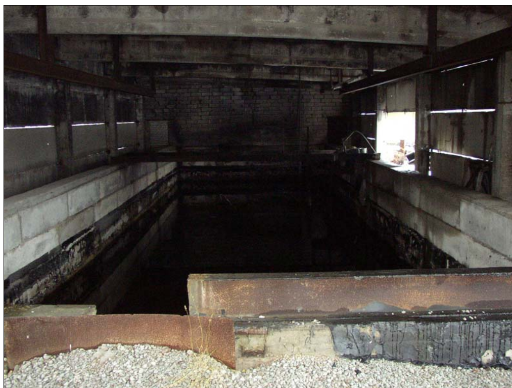
Photo 2500-2. View to naphtha bitumen storage (1); photo 30.10.2002
