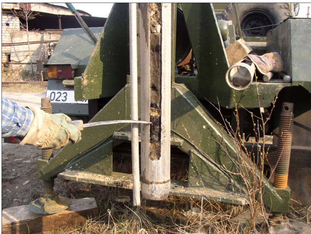
Photo 2410. Bitumen in drilling core bore hole 2410 between 0,7 and 0,8 m
