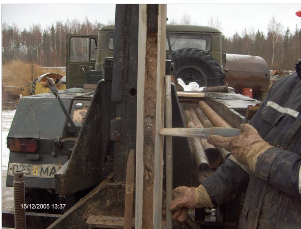
Photo 7309. Oily layer at depth 2,5 m in bore hole 7309
