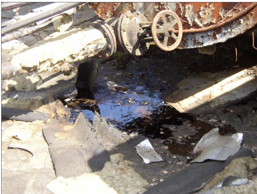
Photo 3406. Spilled black oil in concrete bath under tank 17a
