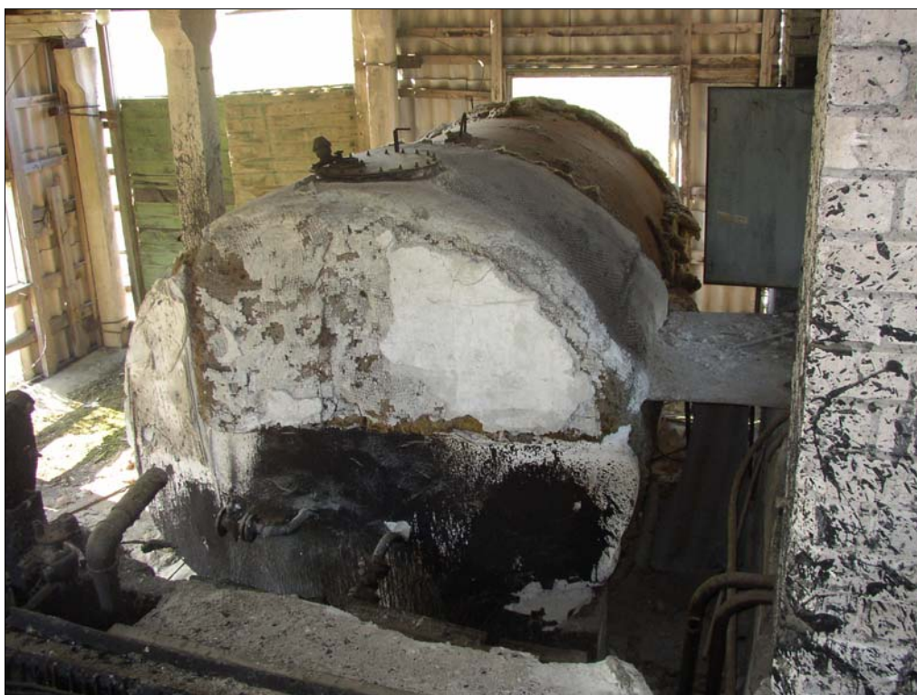
Photo 3402. Tank with kukersool residue inside the roof mastic producing unit
