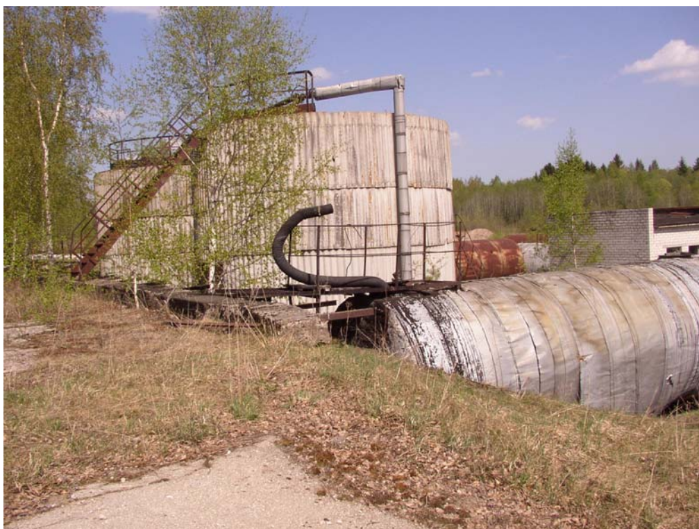
Photo 3408. 200-m 3 tanks 13a and 13b, foreground water tank
