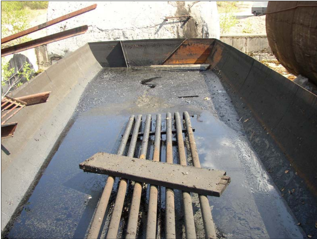
Photo 3405. Half cut tank 17c with residue of black oil
