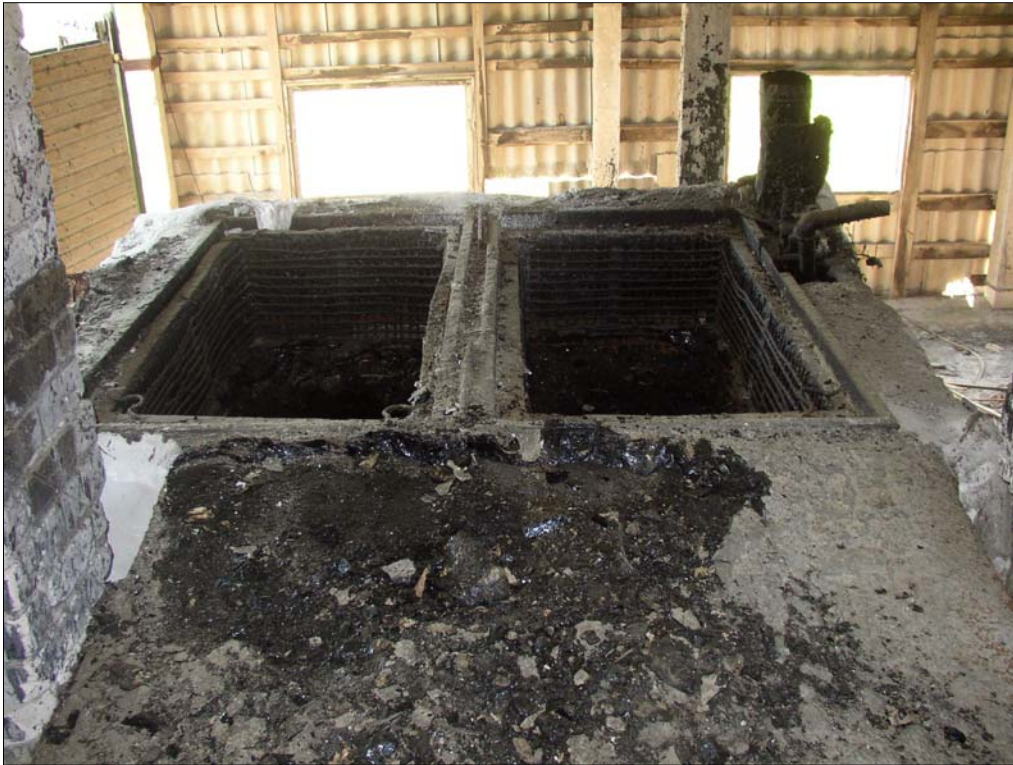
Photo 3403. Boilers inside the roof mastic producing unit
