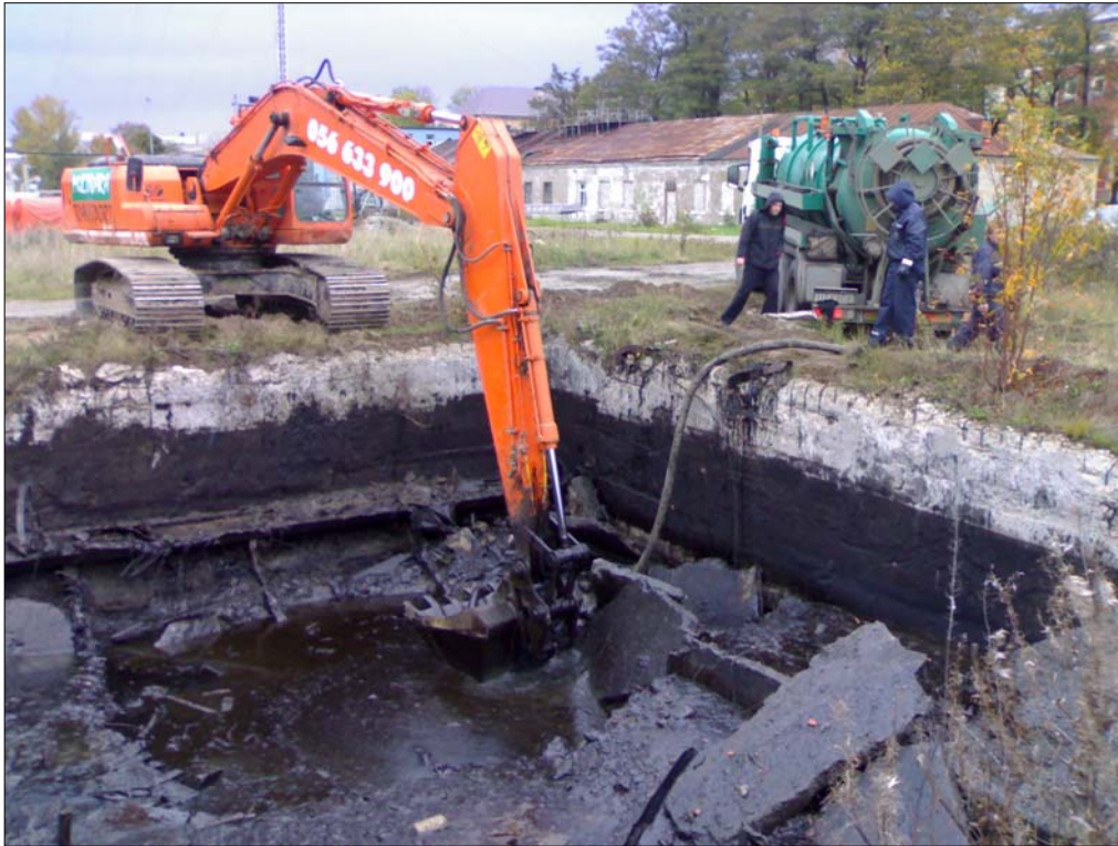
Photo 1500-5. View to cleaning process of the former bilge water separator in year 2006; (Photo from EcoPro report)
