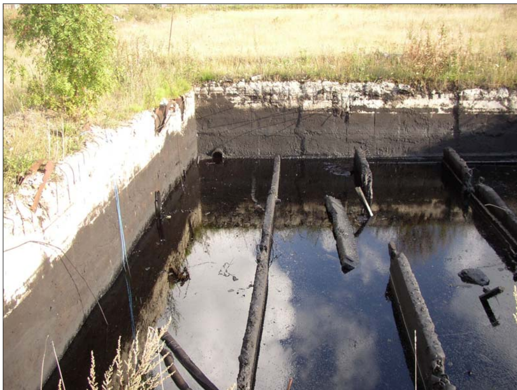
Photo 1500-2. View to the same bilge water separator; in the left farther corner is visible end of pipe, where to can flow also the free phase of oil
